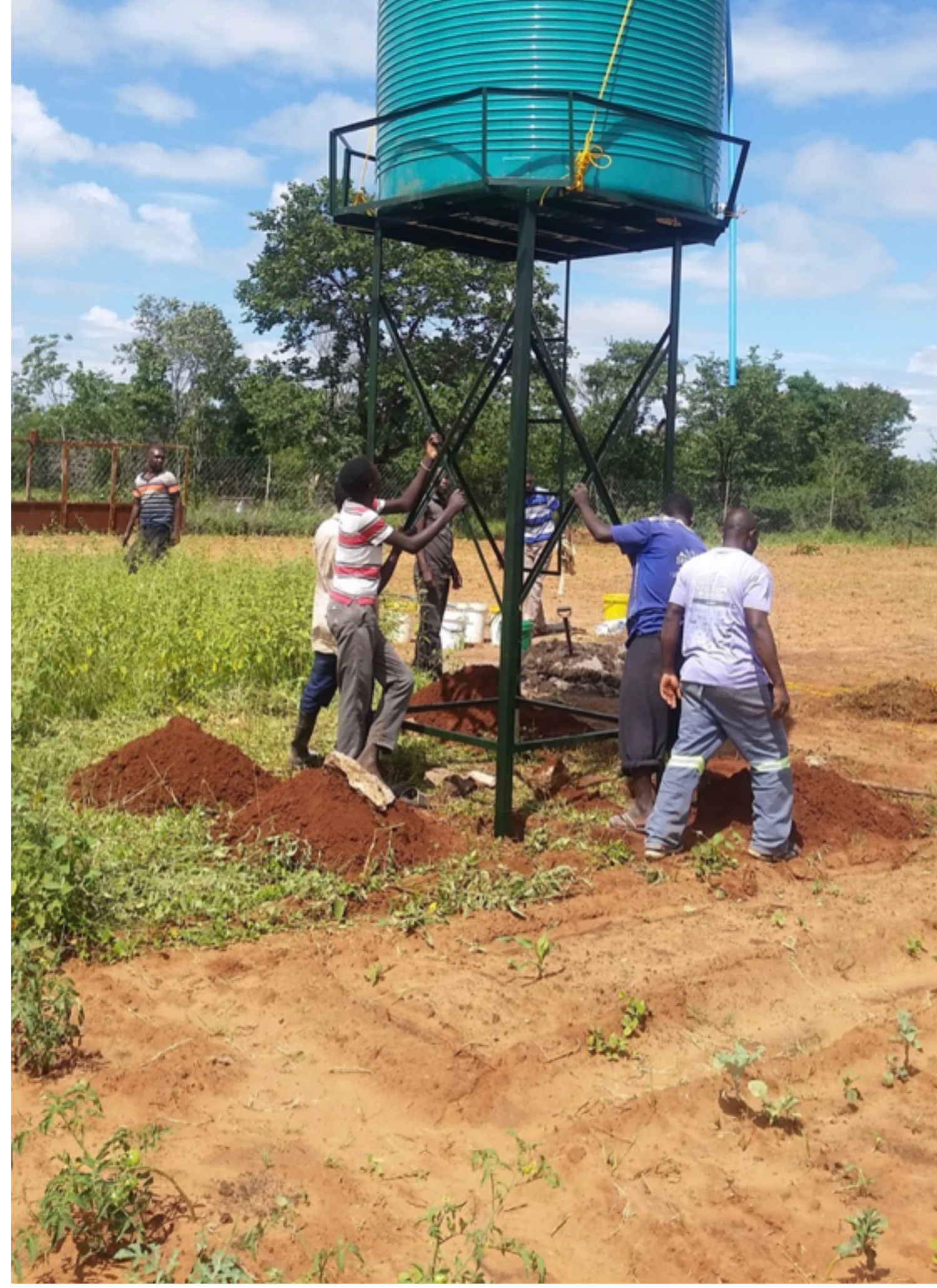
New water tank and vegetable beds set up for a new Community Garden in Chiural Village, Gokwe, Zimbabwe
